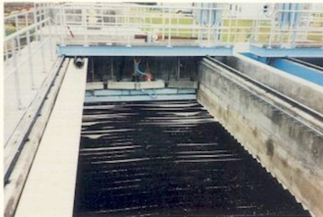
Conventional TBF problem #3—depressions in filter bed indicate media loss through the underdrain
