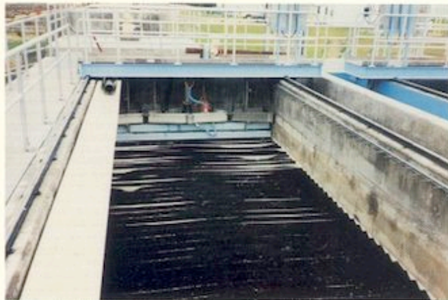
Conventional TBF problem #3—depressions in filter bed indicate media loss through the underdrain
