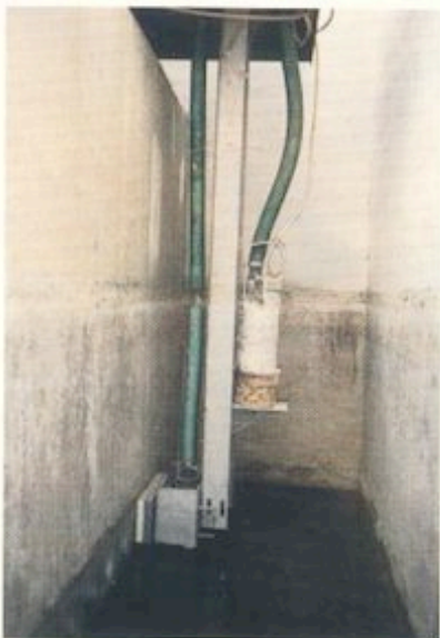
Conventional TBF problem #6—bridge derailment caused by side load on bridge from sliding shoe
