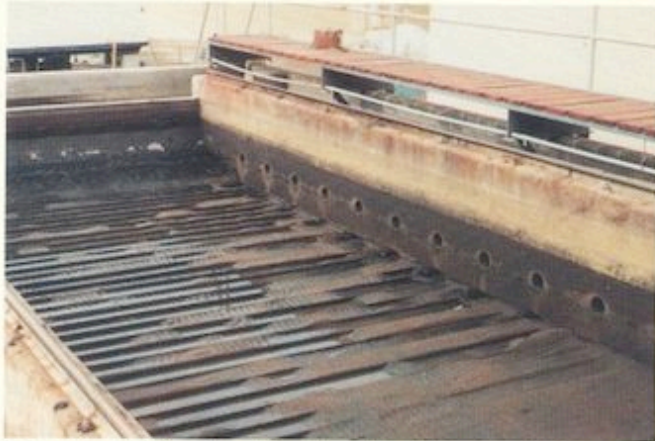
Conventional TBF problem #5—channeling indicates underdrain failure and loss of filter media
