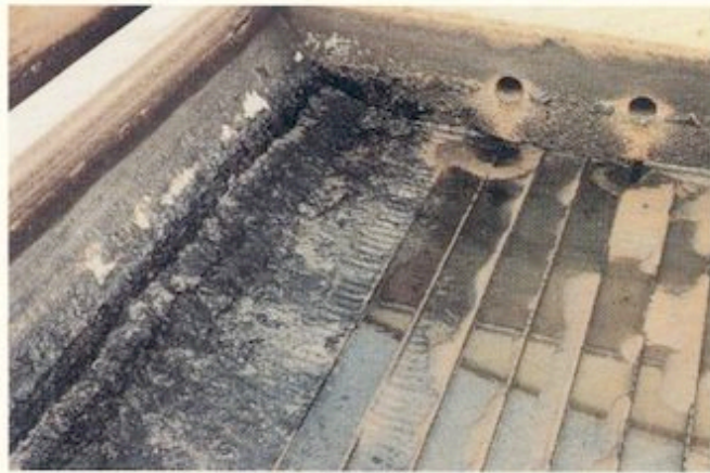
Conventional TBF problem #4—filter media migration to tank ends
