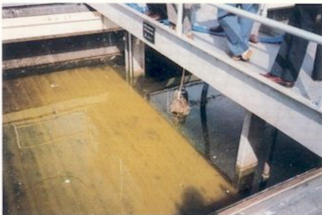
Conventional TBF problem #2—solids accumulation on surface of media means off-line downtime for maintenance
